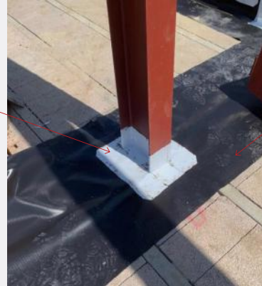
JUTA SELF-ADHESIVE GAS MEMBRANE APPLIED ONTO EDGE OF GP1 AND LAPPED ONTO STEEL & BASE PLATE. NB - GALVANIZED STEEL DOES NOT REQUIRE PRIMER
